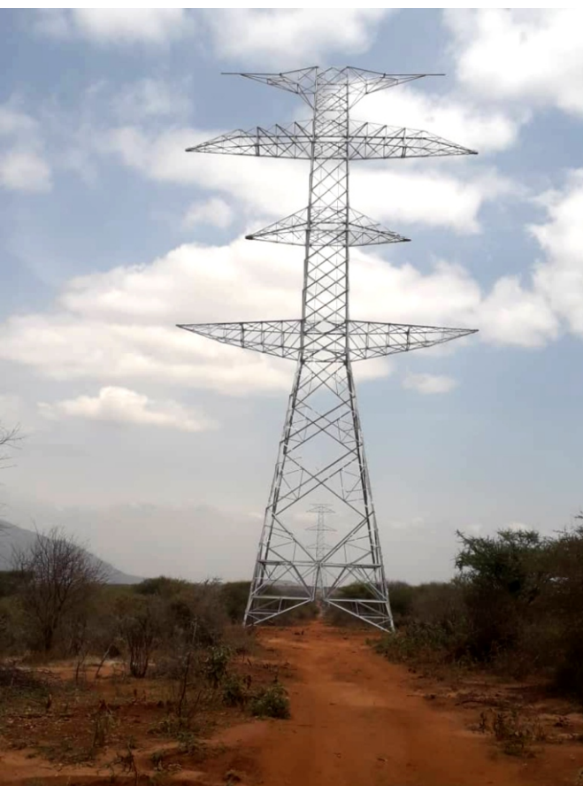
TANESCO - TANZANIA, Turn-key, 114km of 400kV Double transmission line from Namanga (Kenian border) to Substation Lemugur (Arusha)
