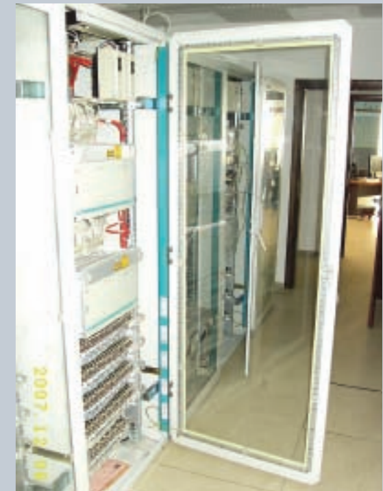
SDH&DWDM Transmission Systems
